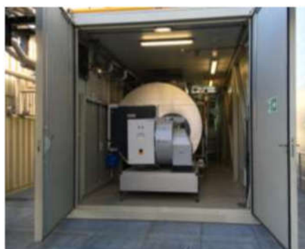
Special Container with Steam Boiler
