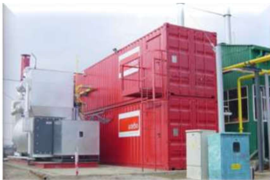
Steam Boiler Plant 6.000 kg/h
