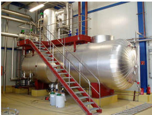
Feed water tank with full degassing
